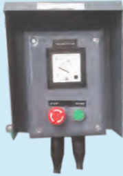
WP Local Control Station
