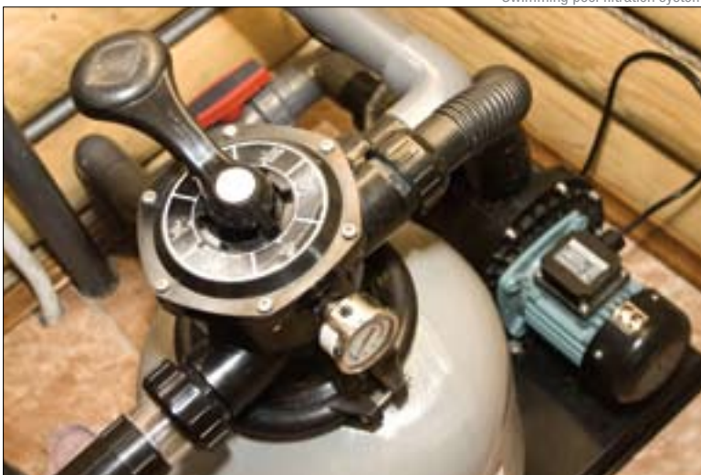
Water filtering system
