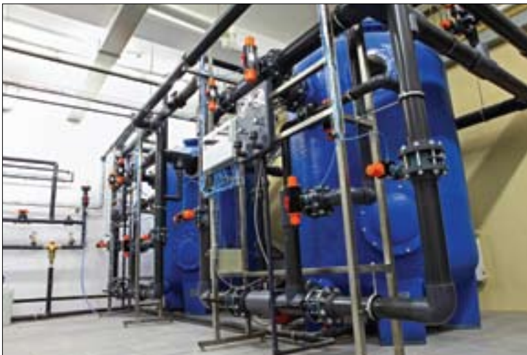
Swimming pool filtration system
